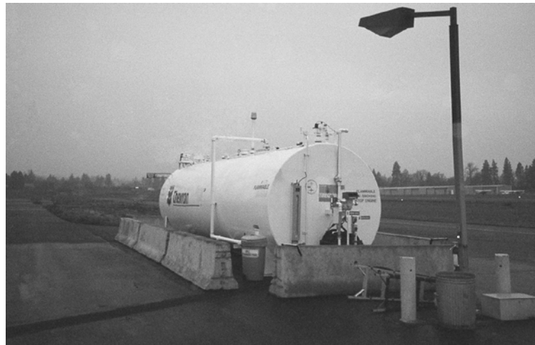
Aviation Fuel Storage (12,000-gallon 100LL AVGAS)
